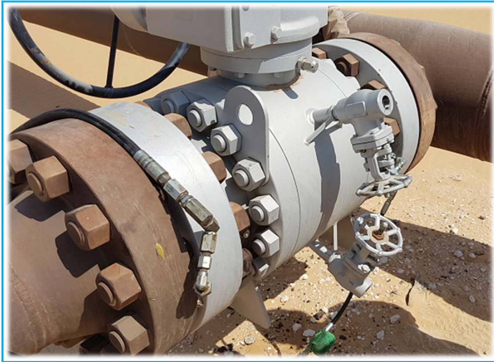
Figure 8: Seat cleaning & greasing application over ball valve
