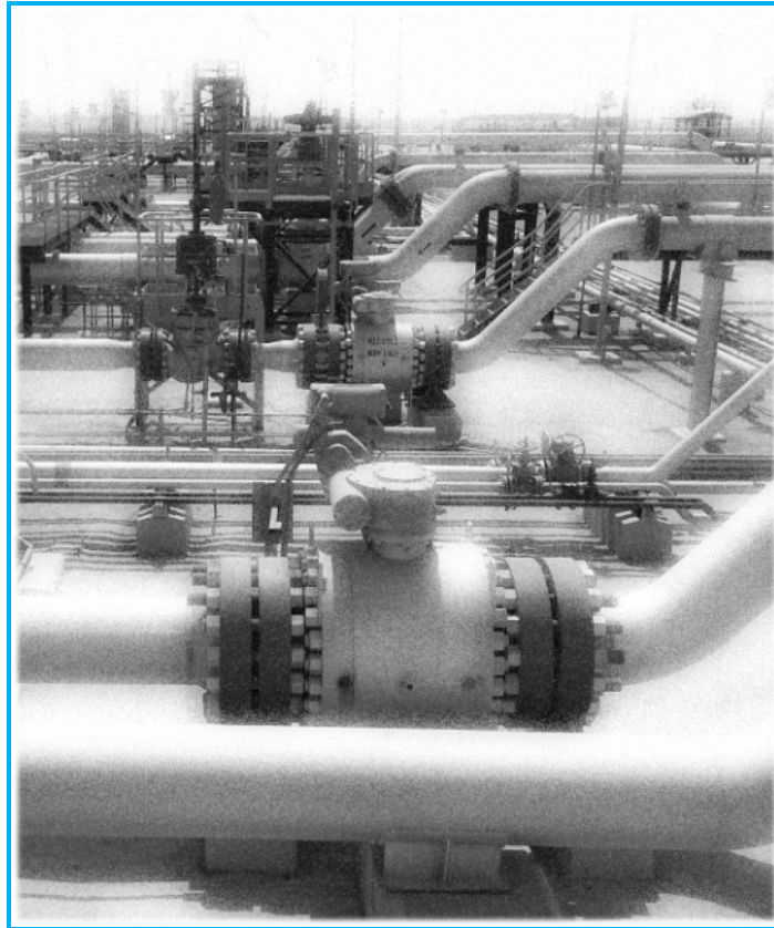
Figure 4: Interchangeable valves at SWID facilities
